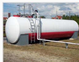
Fuel / Oil Tank Level
